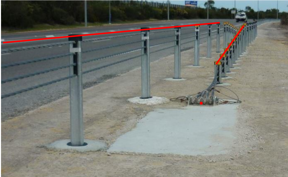
Figure 8j – Re-directive, wire rope, tapered to ground leading end. Wire, rope barrier with plastic top material on steel uprights.
