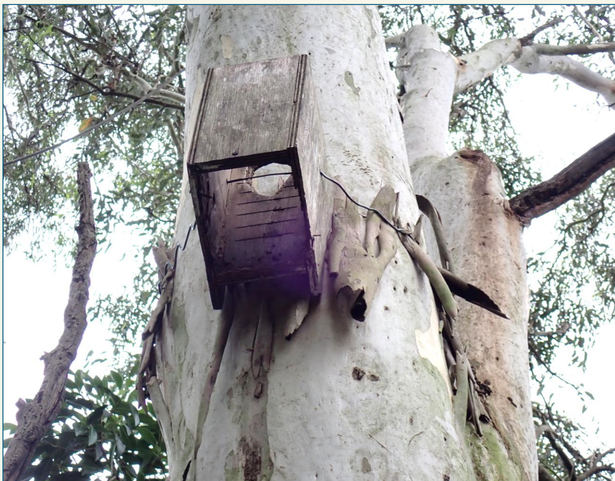
Older style timber Nest Box 1221 at Wynnum North Road is dilapidated and unable to support native wildlife..
