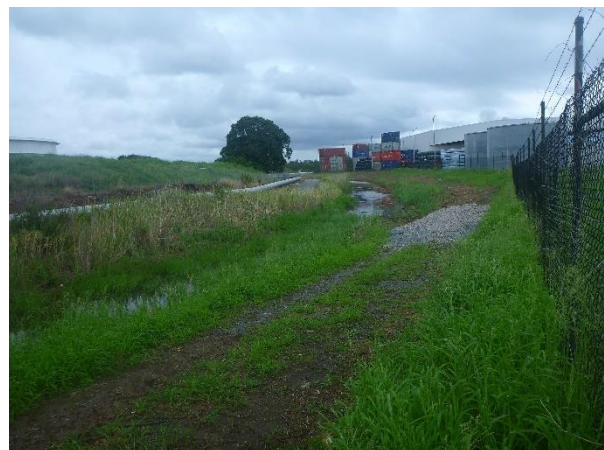
Figure 3-4 Port Gate Drain
