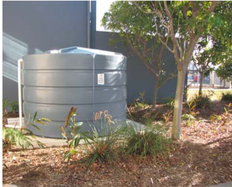
Rainwater tank at Port Office
